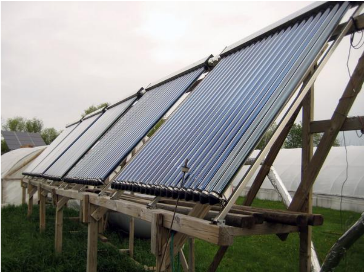
Evacuated tube solar thermal system at Appleton Farms, a property of The Trustees of Reservations in Ipswich, MA
