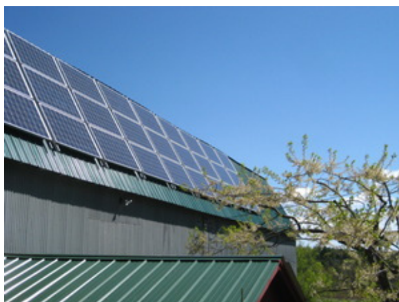
Solar panels on barn roof
