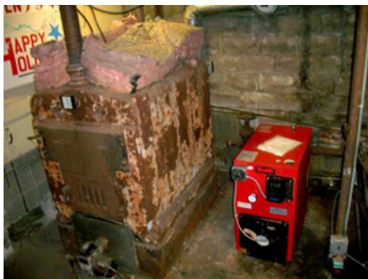
Old and new boilers at Dutchies Greenhouse in Plymouth, Mass.
