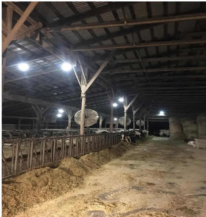
Energy efficient lighting at Catlin Farmstead in Winchendon. This lighting upgrade saves over 5000 kWh annually.
