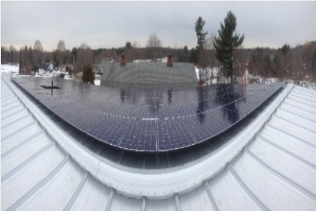
Roof mounted solar array at Farmer Dave's in Dracut. This array generates over 30,000 kWh per year.
