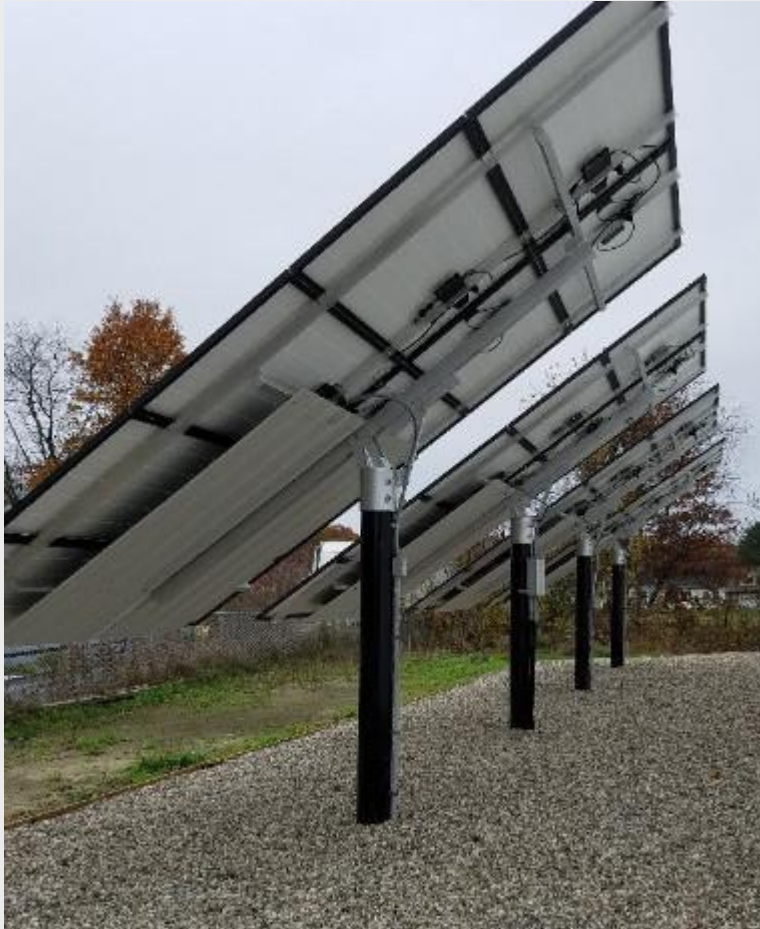
Solar electric array at Honey Pot Farm in Hatfield.
