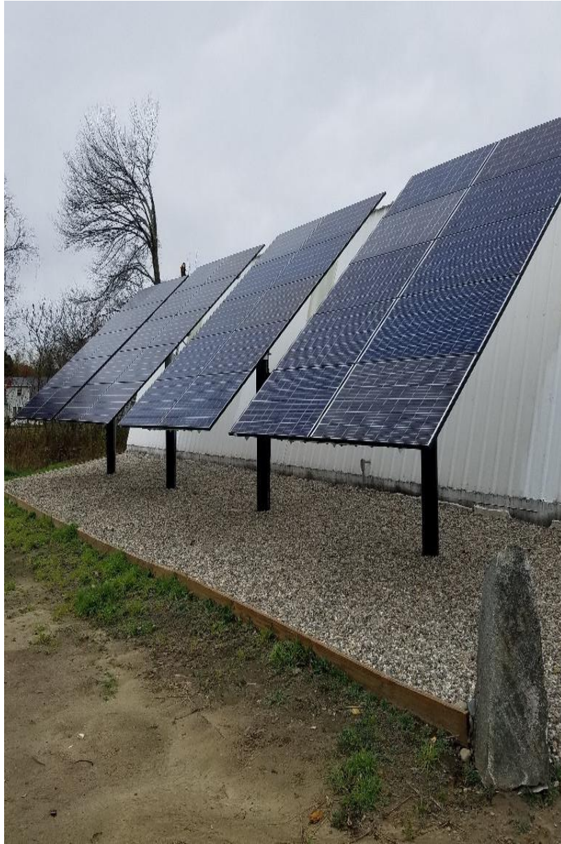
Solar Electric array at Honey Pot Farm in Hatfield.
