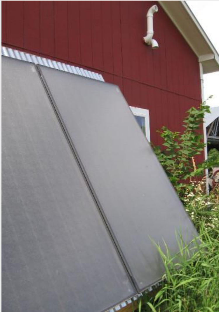
Solar thermal system at Morning Dew Farm in Worthington
