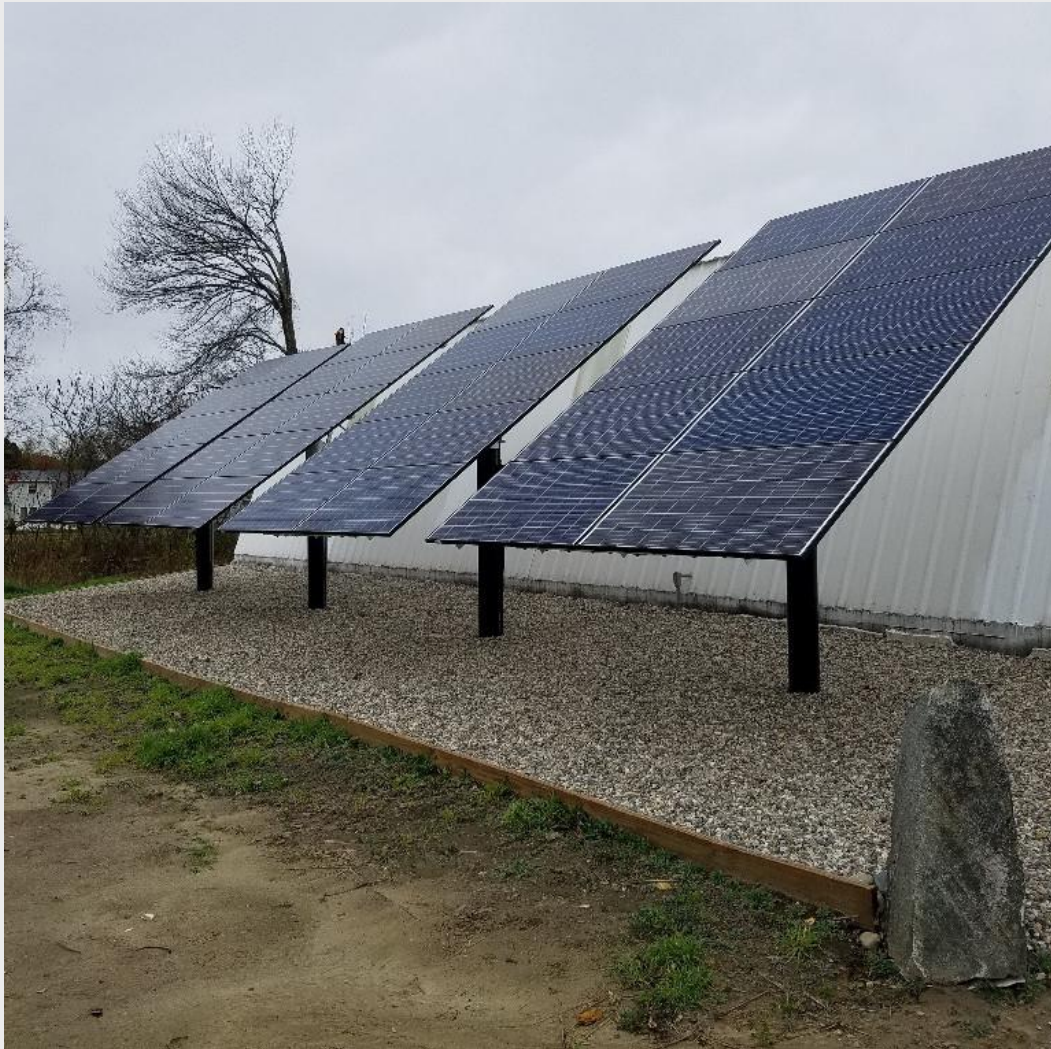
Ground mounted solar electric array at Honey Pot Farm in Hatfield, a 2017 REAP Grant recipient
