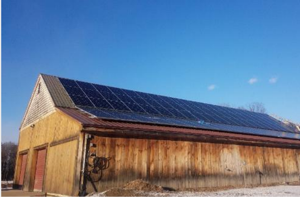
Solar electric array at Mountain View Farm in Easthampton
