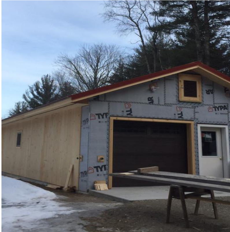
Newly constructed zero net energy maple kitchen at Justamere Tree Farm in Worthington
