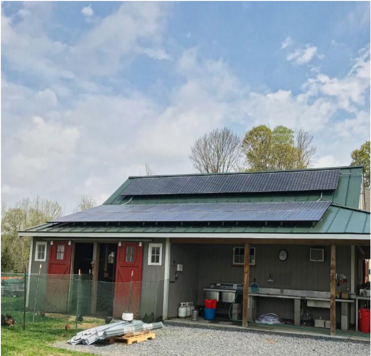
Roof Mounted Solar Electric Array at Red Shirt Farm in Lanesborough
