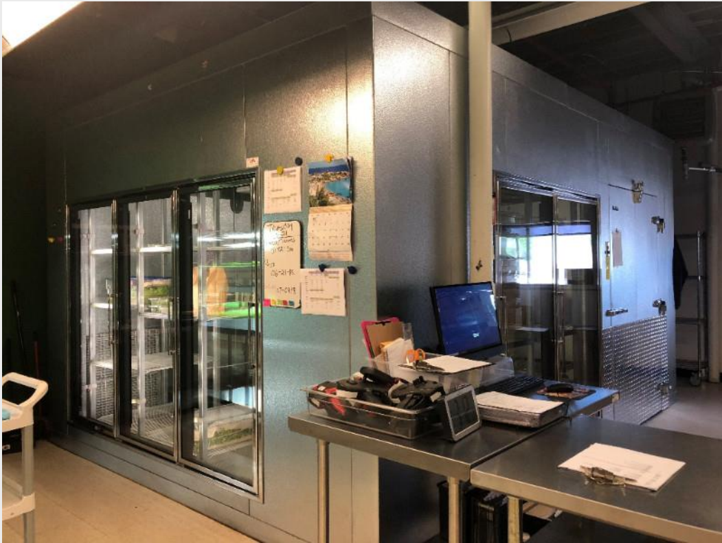
Energy Efficient Refrigeration at Two Friends Farm in Attleboro. This project was completed with the help of an MDAR Special Projects Grant.
