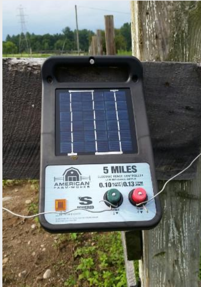
Solar powered electric fence charger at Craig Memorial Equestrian Center in Leverett. This project was completed with assistance and funding from the Massachusetts Farm Energy Program.
