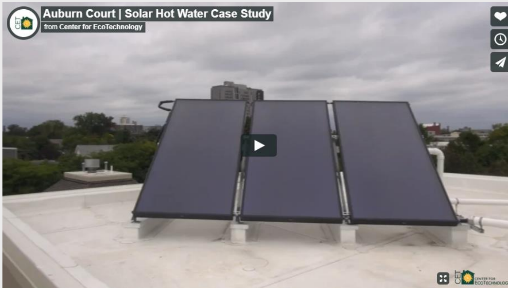
Solar hot water array on the roof of a building in Cambridge. Click the video above to watch a brief case study about solar hot water, and learn about some of the applications and available incentives for this technology!
