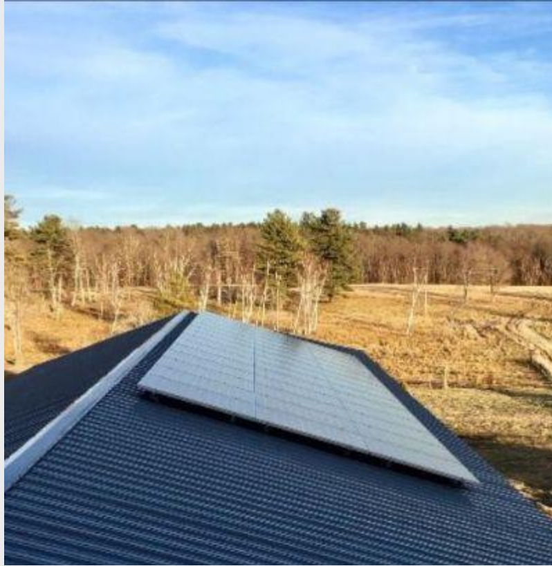
Roof mounted solar electric array at Maple Hill Farm in Hardwick. This array produces over 17,000 kWh annually.
