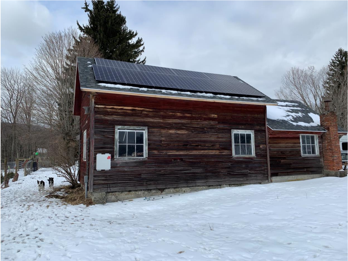
Roof mounted solar electric array at Maybrook Farm in Pittsfield.
