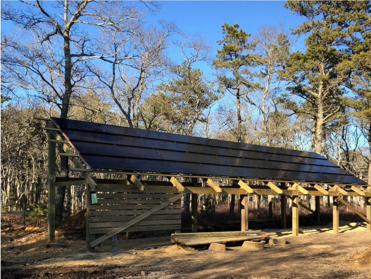
Ground mounted solar electric array at Pleasant Lake Farm in Harwich.
