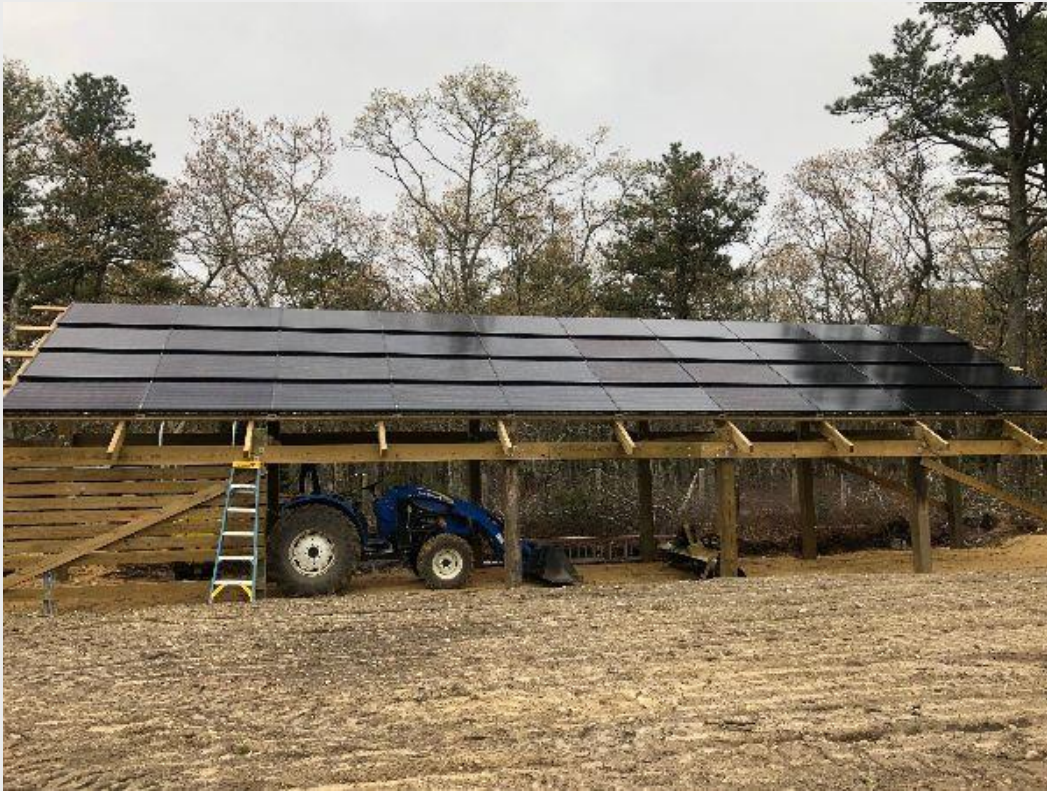
In-progress ground mounted solar electric array at Pleasant Lake Farm in Harwich. Keep reading for more information on this project!
