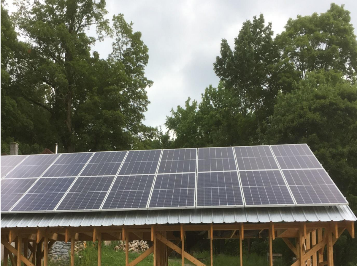
Roof mounted solar electric array at Sawyer Farm in Worthington.
