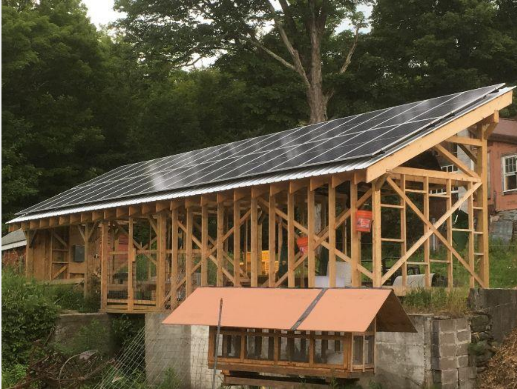
Roof mounted solar array at Sawyer Farm in Worthington. Keep reading for more information on this project!
