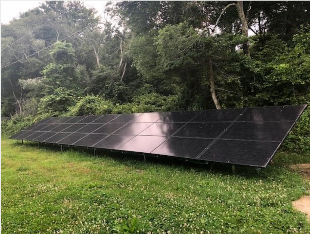
Ground mounted solar array at Ivory Silo Farm in Westport. Keep reading below for more details about this renewable energy project!
