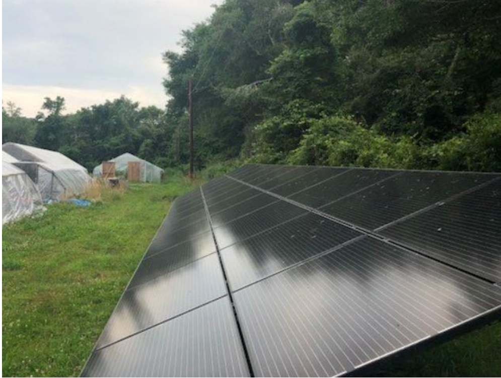
Ground mounted solar electric array at Ivory Silo Farm in Westport.
