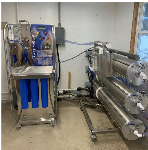
New reverse osmosis system at Round Mountain Sugarhouse in Northfield.
